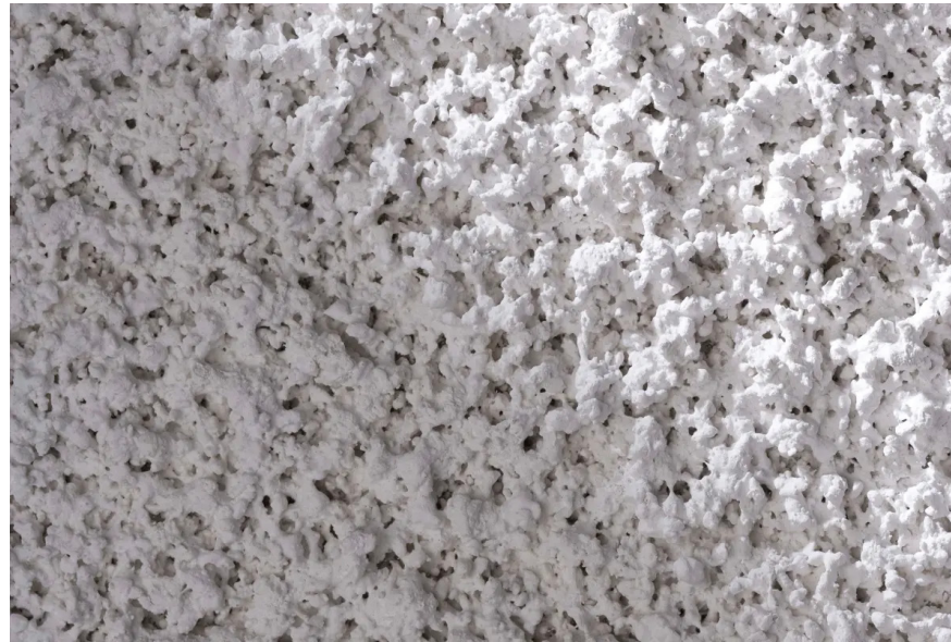
Acoustic plaster wall
